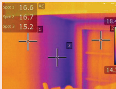
Thermal image of cold window reveal at The Old Farmhouse
